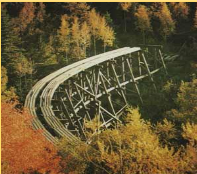
Mexican Canyon Trestle For 50 years the Alamogordo-Sacramento Mountain Railroad carried passengers and freight from the desert floor into the tall pine country of Cloudcroft, climbing 6,000 feet. The train line was abandoned in 1948.
