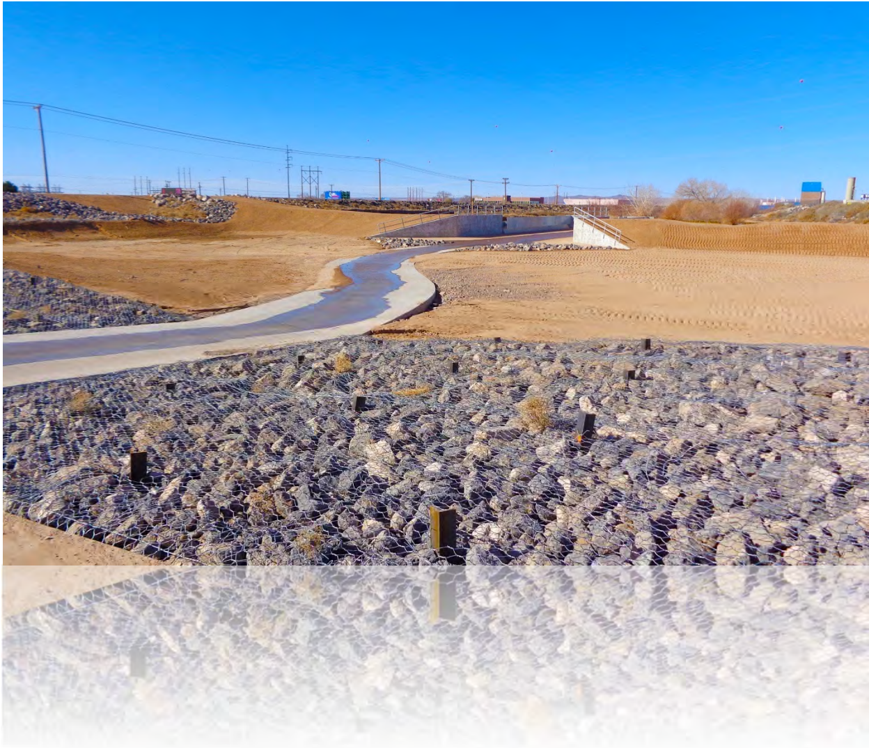
A regional water quality structure was built in connection with the I-25/Paseo del Norte Interchange Reconstruction
