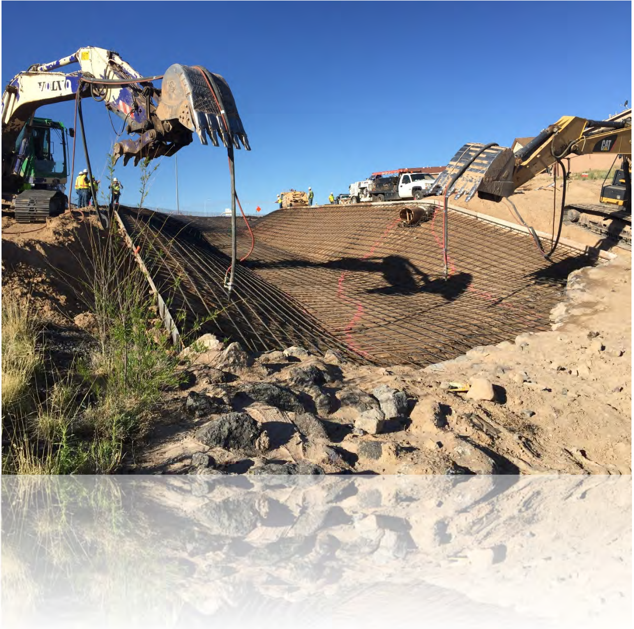
The first day of shotcreting in April 2017 on the West I-40 Phase IV project
