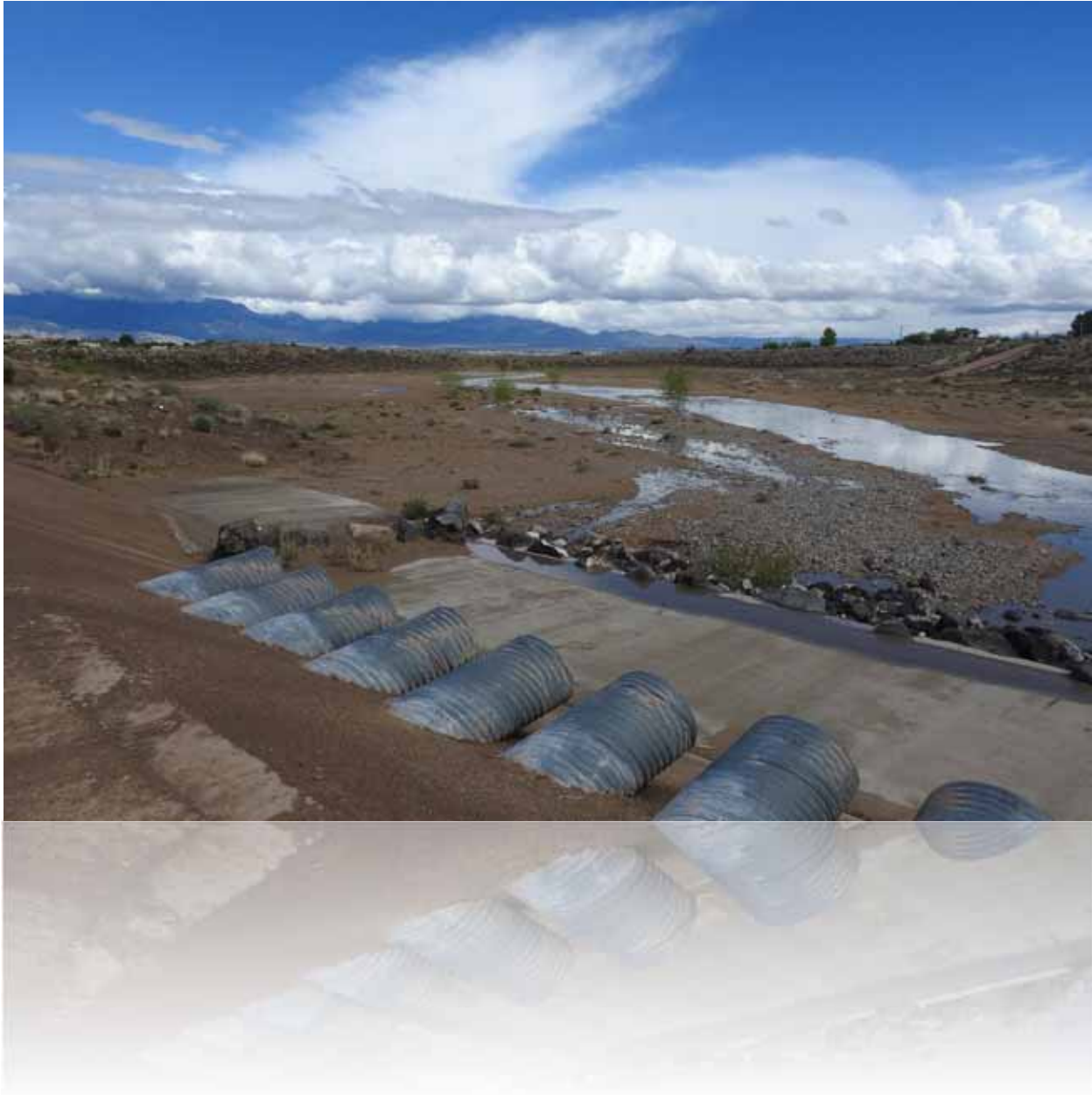
Black Dam water quality structure
