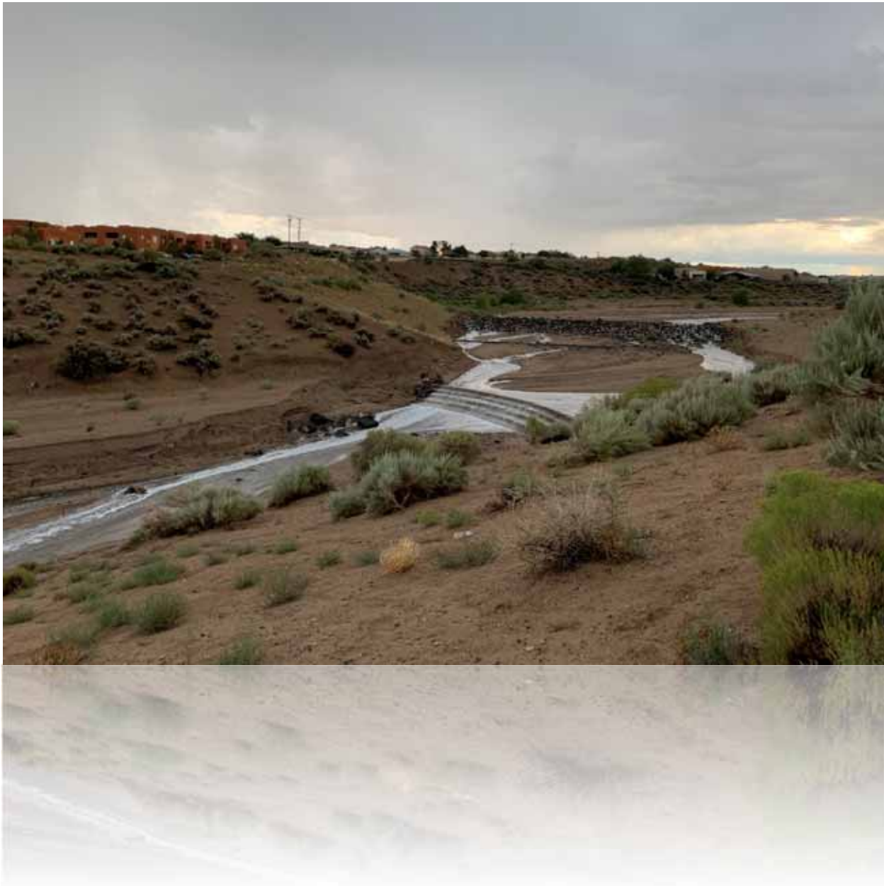
Storm flow running down the Calabacillas Arroyo over Grade Control Structure 7a
