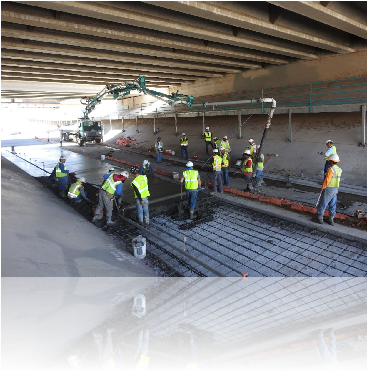
Contractors utilizing a concrete pumper truck to complete overlay of the North Diversion Channel
