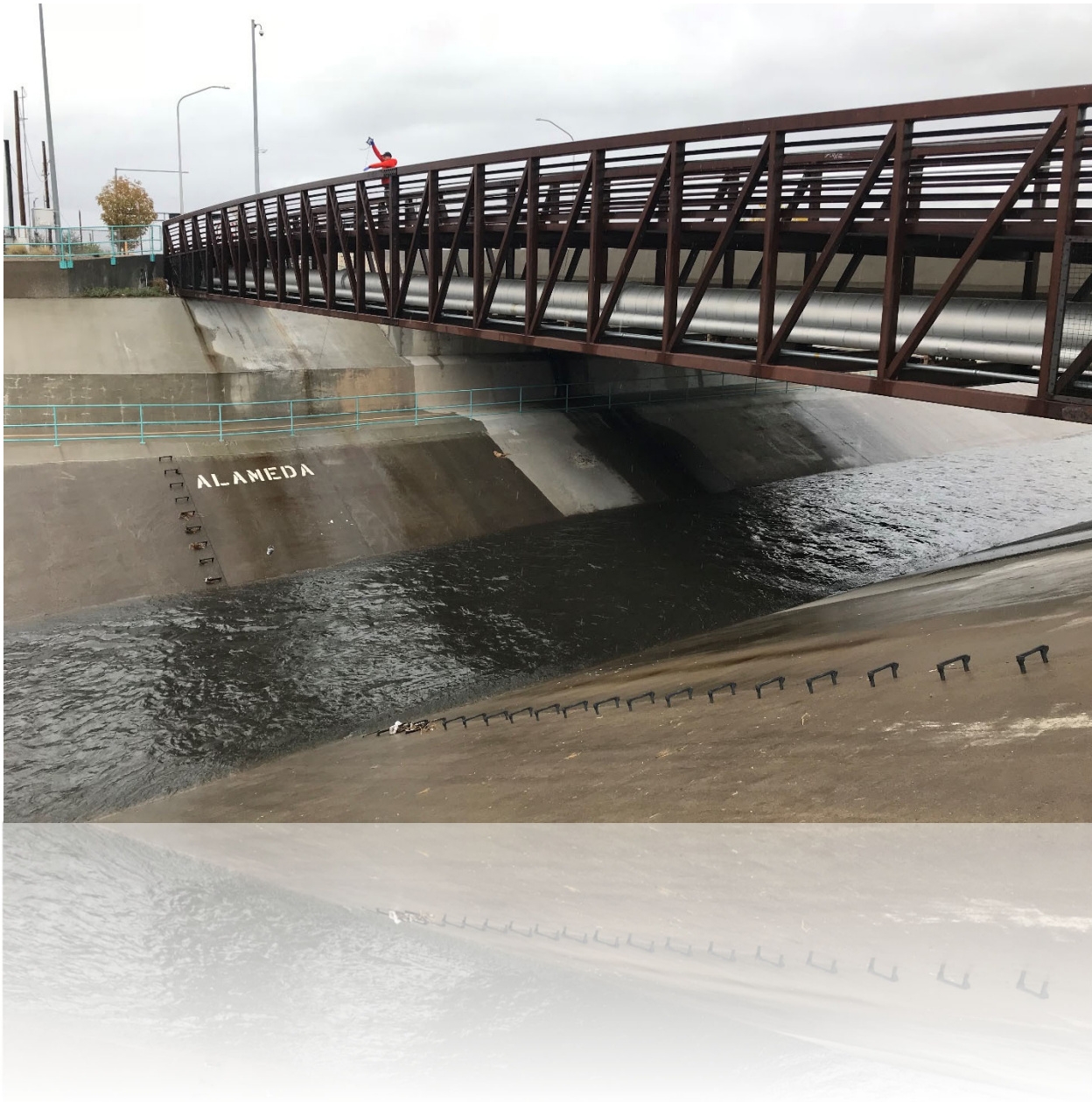
A small rainstorm travels down the North Diversion Channel at Alameda Road
