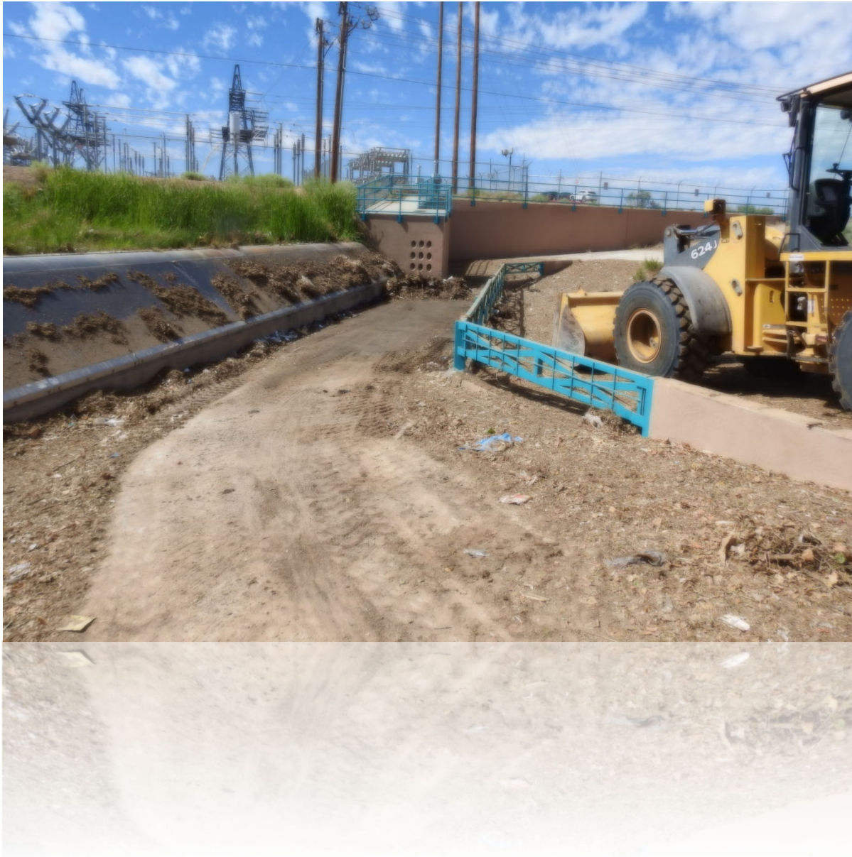
Maintenance crews clean out the Vineyard Water Quality Structure that keeps debris from entering the Rio Grande
