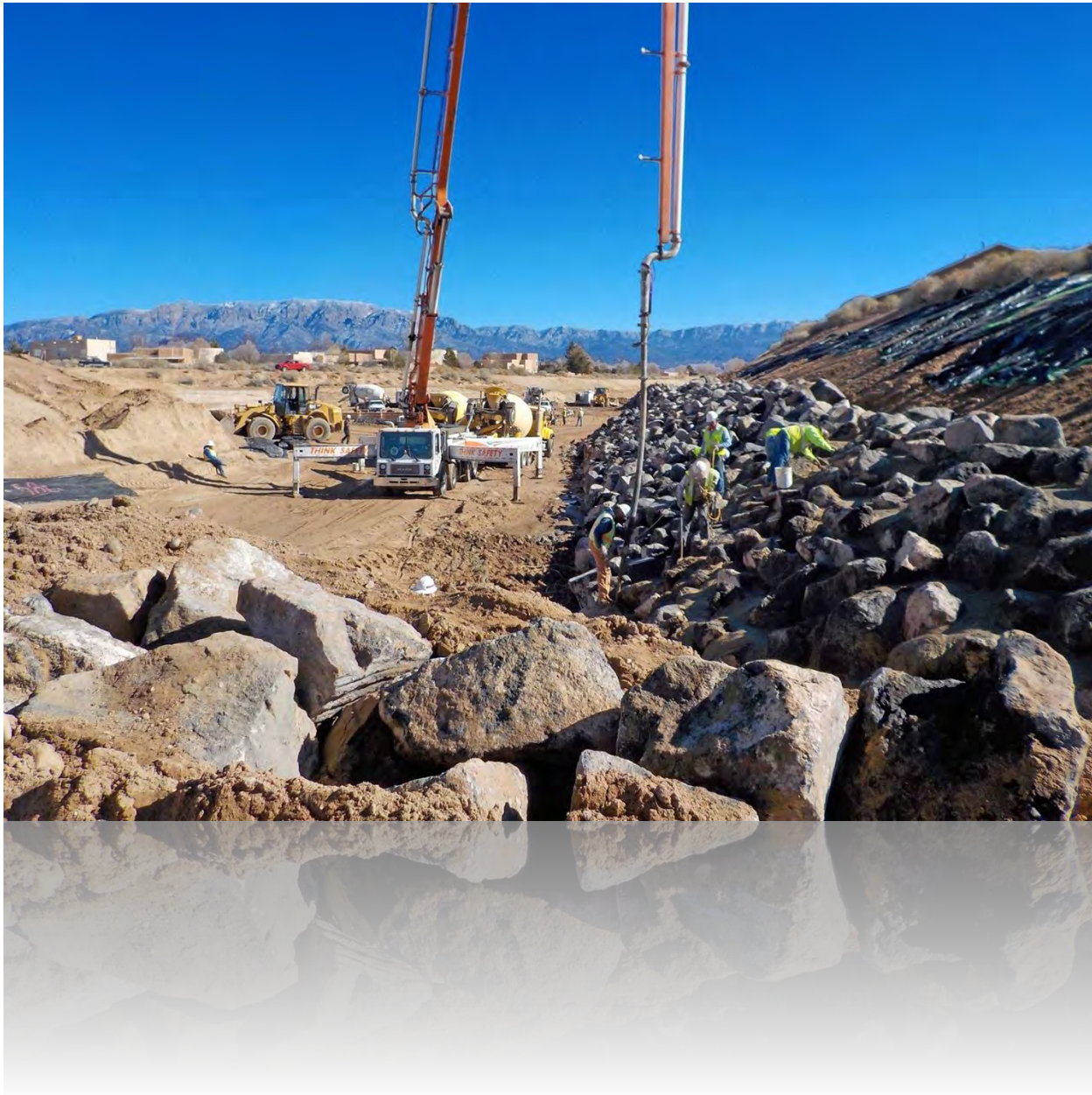
Grouted boulders provide naturalistic bank protection for arroyos in the Albuquerque area
