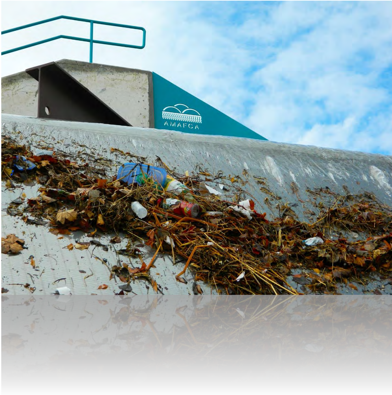
Water Quality Structure capturing debris
